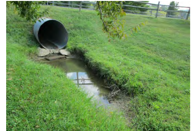
Standing water at pipe under Park Road crossing
