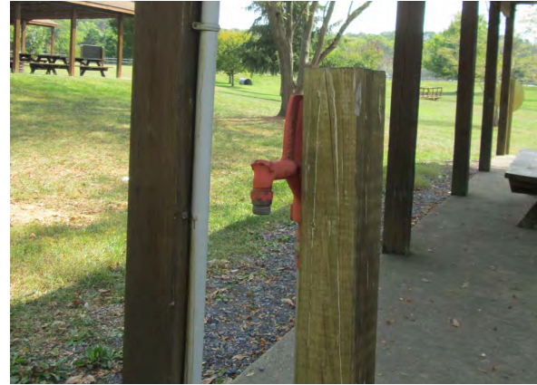
Water connection at the Kiwanis Park Shelter
