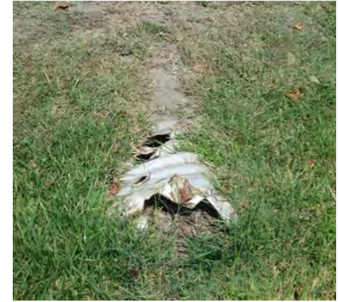
Clogged drain pipe under Park Road
