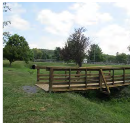
Pedestrian bridges not ADA accessible
