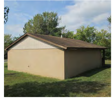
Entrance to restroom obscured
