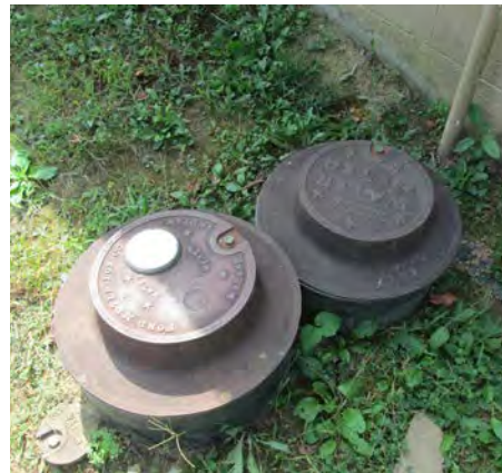
Water meter at restroom facilities
