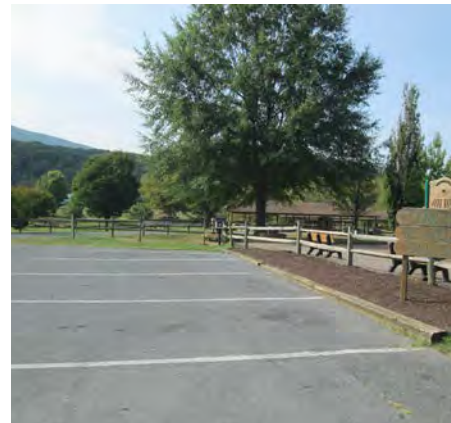
No accessible parking at playground
