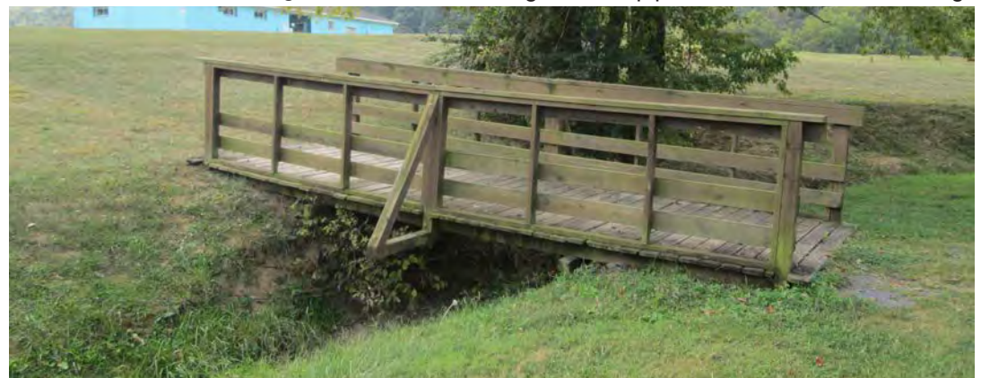
Stream banks eroding at pedestrian bridge location
