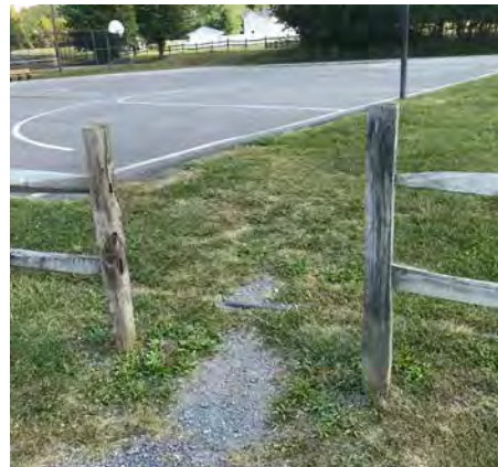
Courts are not served by accessible routes that connect feature with accessible parking space
