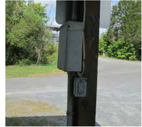
Electric at the First Bank Park Shelter
