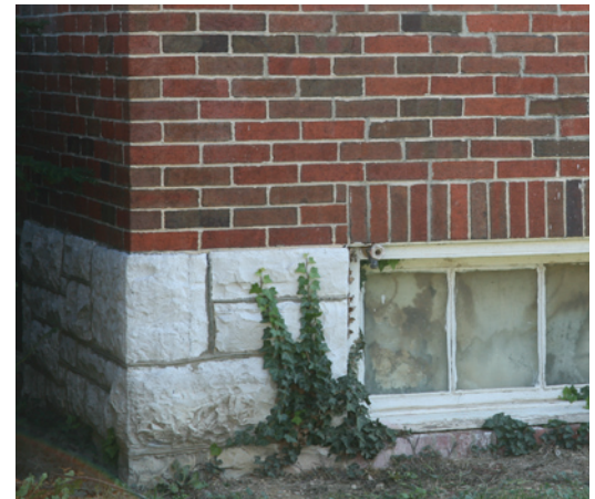
It is best to keep vegetation clear of the foundation as roots may leach nutrients from the mortar.
