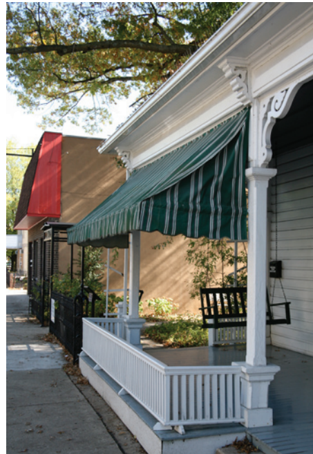
The awning on the porch of the Strasburg Library is properly attached under the cornice.
