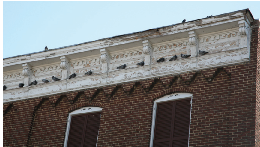
A wooden cornice with Italianate details sits above a brick pendant cornice.
