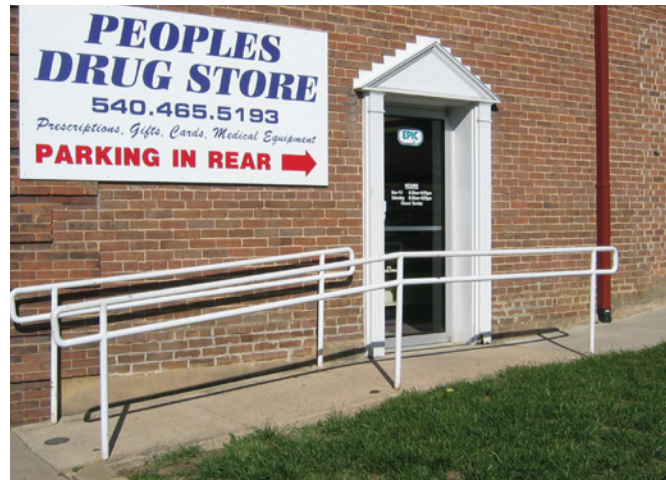
A pipe railing is located to each side of the ramp that provides handicap access to the side entrance of the drug store.
