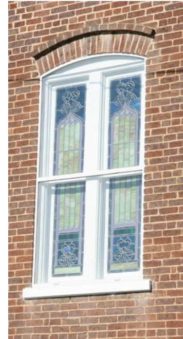
The segmental arch associated with arched window openings embellished in this example by a projecting course of header bricks.
