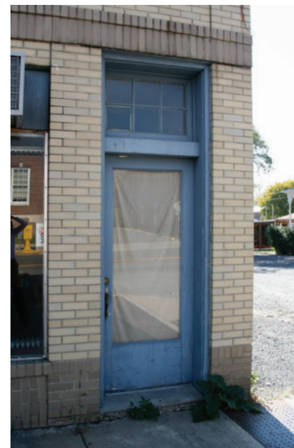
A fully glazed door with a six-light transom was used for a secondary entrance at the Strasburg Theater.
