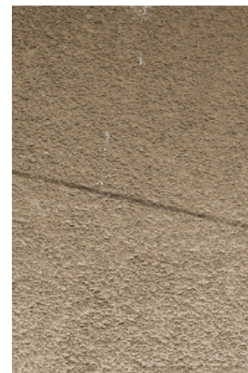
Rough-finished stucco is often associated with the Arts and Crafts movement and is seen on Bungalow and American Foursquare houses in the district.
