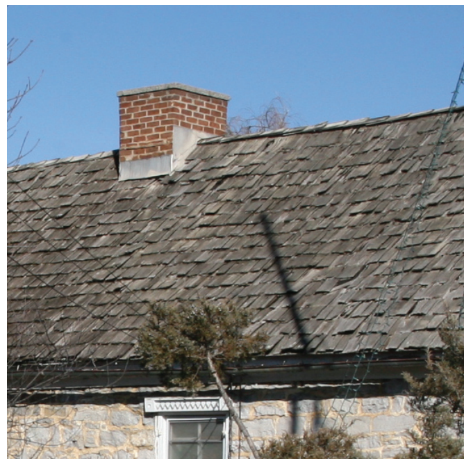
The Frontier Fort roof is currently covered in non-historic wood shingles.
