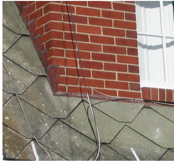
The diamond pattern of this shingle is usually associated with cement-asbestos shingles.
