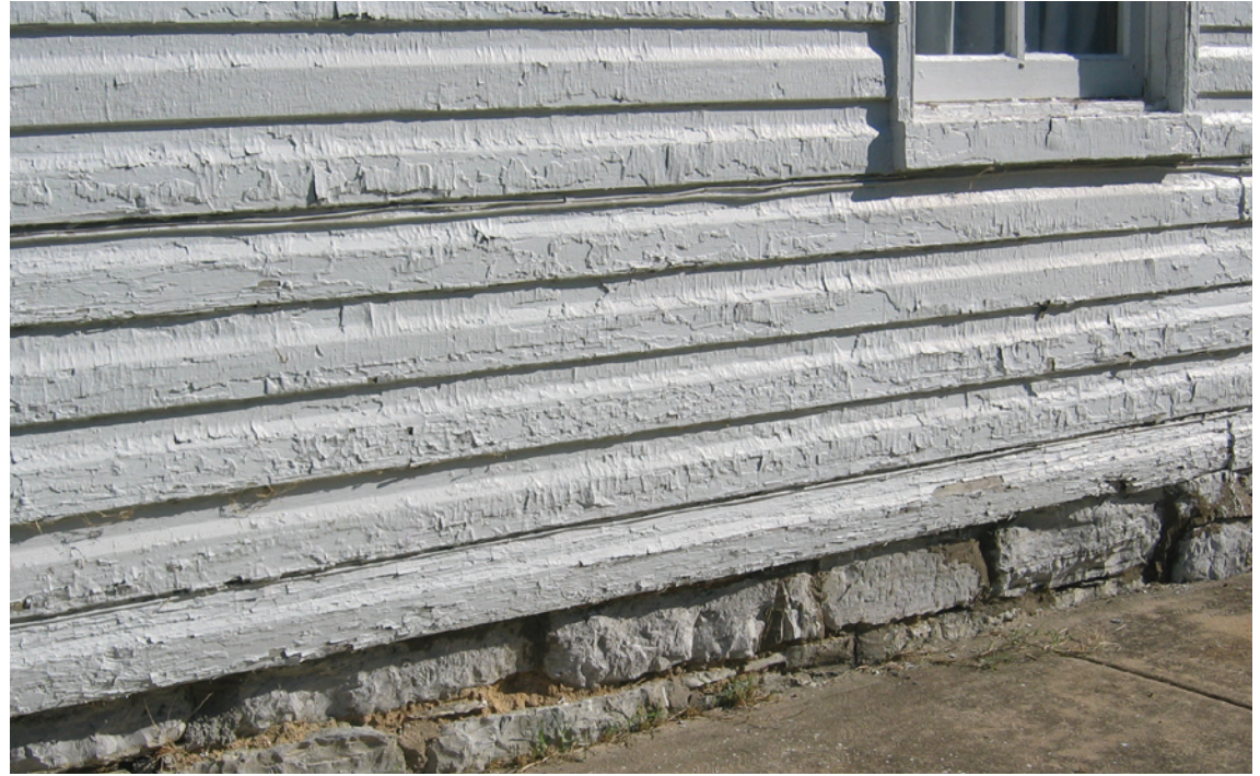
Layers of accumulated paint over time may lead to an uneven surface appearance and paint failure.
