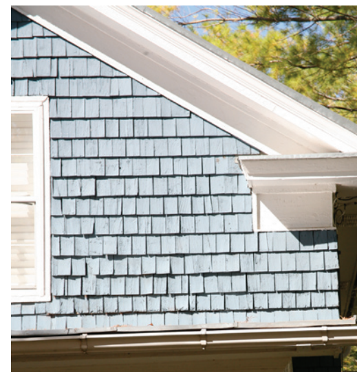
Wooden shingles as a wall cladding material gained popularity in the late nineteenth century.
