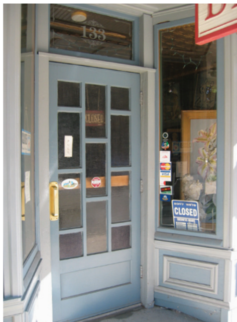
Note the offset pane divisions on this storefront door on King Street.
