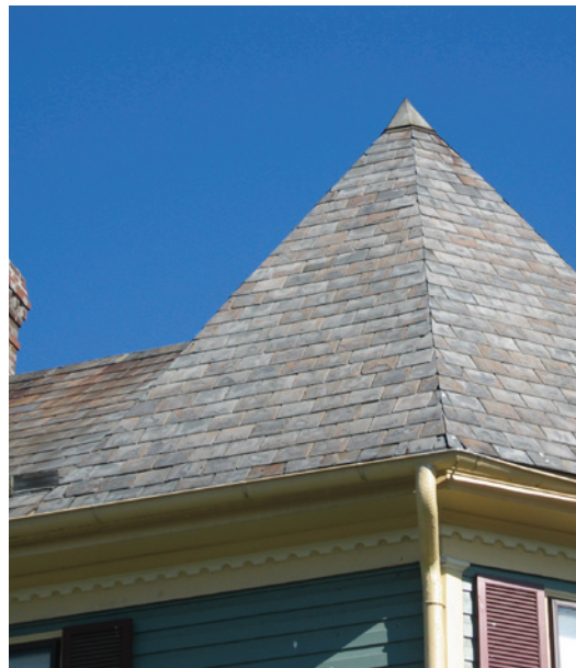
The subtle variations in the tone of this slate and its apparent good condition may indicate that this roof is clad in Vermont slate.
