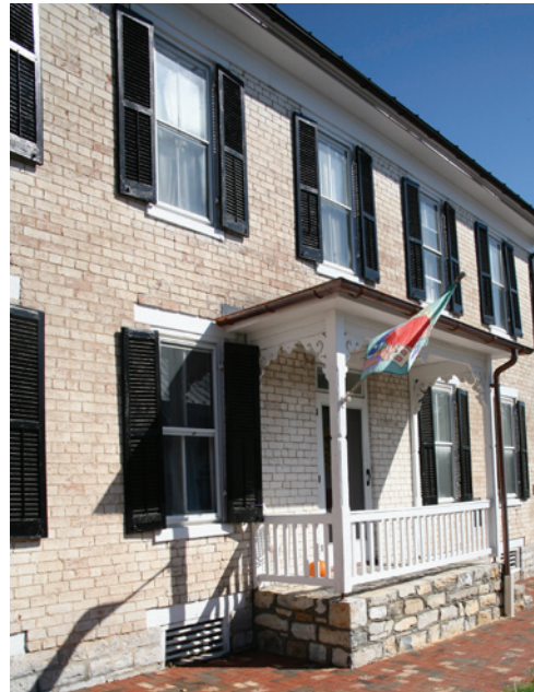
A Victorian one-bay porch is a later addition to this Greek Revival residence.
