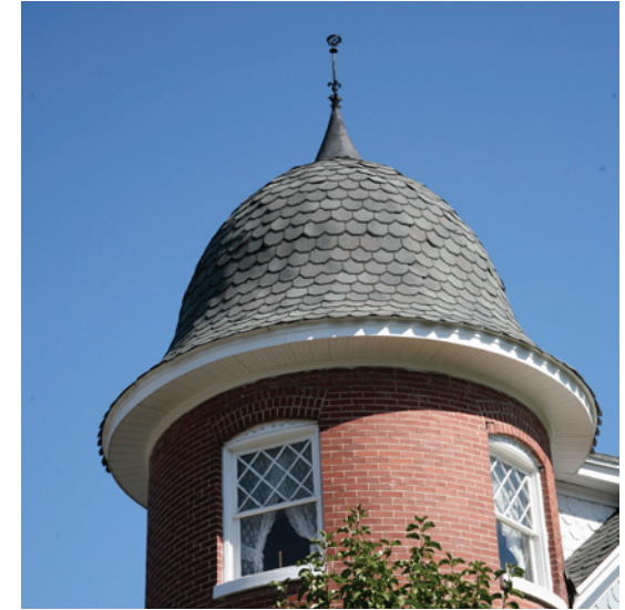
Asphalt roofing products that simulate slate can be found in the district and may allow the flexibility to cover curved surfaces such as this turret.
