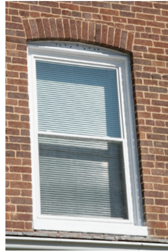
While the opening is arched, the glass panes of this one-over-one window are square; the wooden frame fills the arch with a carved panel.
