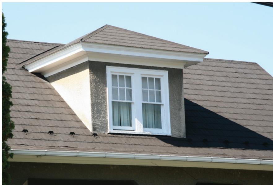
This stucco clad dormer has a hipped roof covered in metal shingles and provides light to the upper level of a Bungalow in the district.
