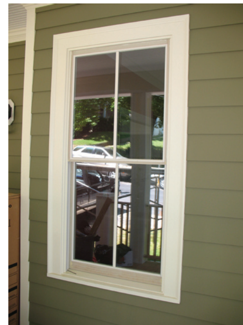
A simulated divided light window is shown here trimmed in a composite material. The architrave molding of the trim replicates a historic profile.
