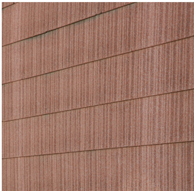
The texture and striations of this wall cladding identify it is an asbestos shingle product.
