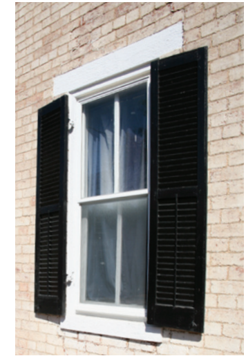
This window has a lintel that extends past the opening, common in Greek Revival architecture.
