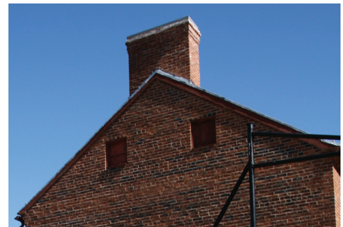
Located entirely within the end wall of the building, this chimney reflects advancements in technology that allowed interior chimneys to become possible in the early nineteenth century.
