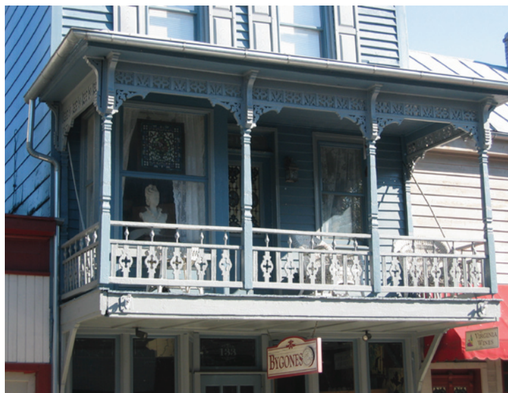
Second-story gallery porches are a character-defining feature of the commercial portion of the Old Strasburg district.
