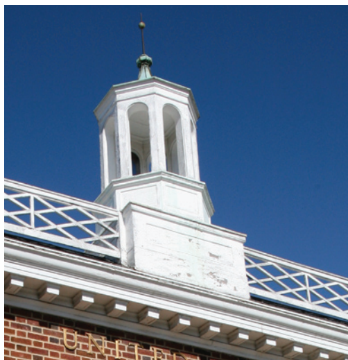
A cupola is located behind the gallery balustrade on the roof of the Strasburg Post Office and is capped by a copper roof and finial.
