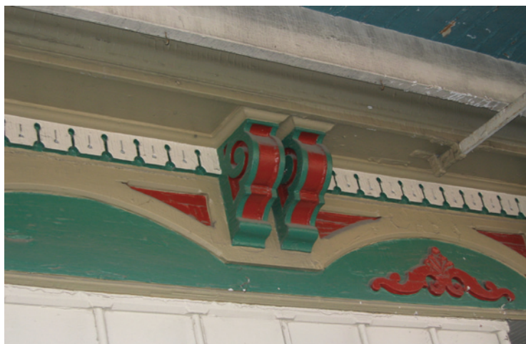
When decorative wooden trim is well-maintained and painted in appropriate historic colors, it adds a character-defining element to a storefront.
