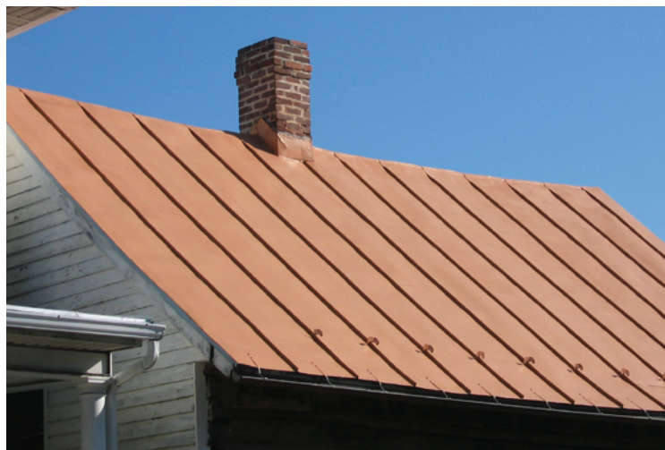
Standing-seam metal roofs need to be kept painted to prevent deterioration.
