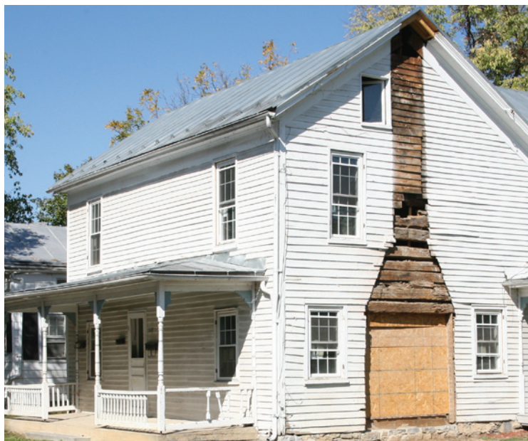
Rehabilitation work on this historic residence included the removal of the exterior chimney and reveals an apparent log structure to which a second story was later added. The outline of the lower portion of the chimney and its exterior placement likely date the original portion of the house to the early nineteenth century.
