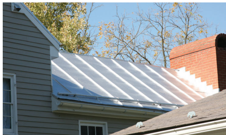
A new galvanized standing-seam metal roof often needs to weather before paint will adhere properly.
