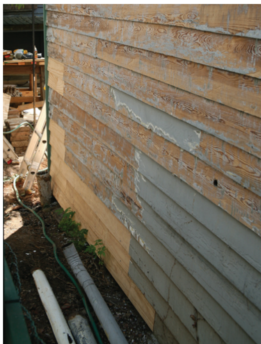
Preparation for painting has begun. Much of the old paint has been scraped to a sound layer and clapboards beyond repair have been replaced in kind.
