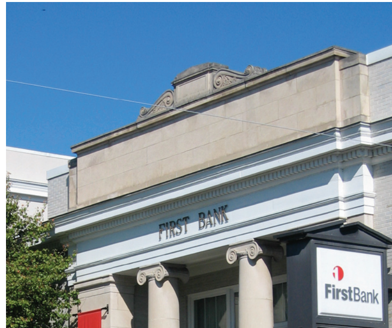
Classical cast stone decorative elements adorn the brick parapet of this bank building on King Street.
