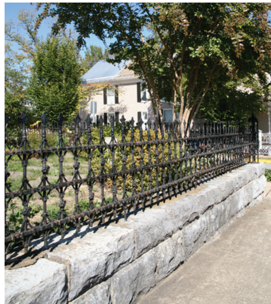
In some instances, a cast iron fence is mounted on top of a low stone wall.
