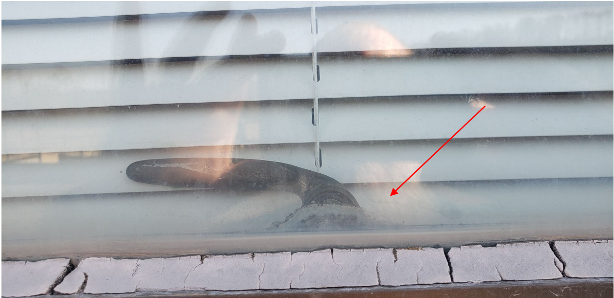
Figure 7 Frosting inside the panes, seals bad
