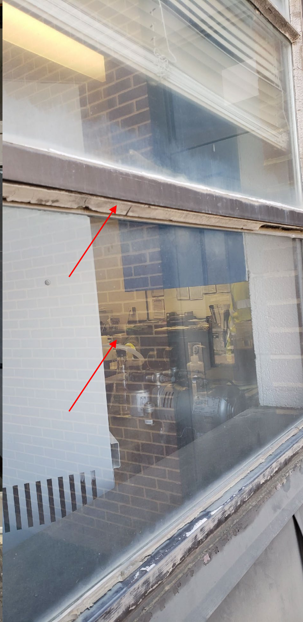
Figure 5 Grout missing and one pane of glass missing
