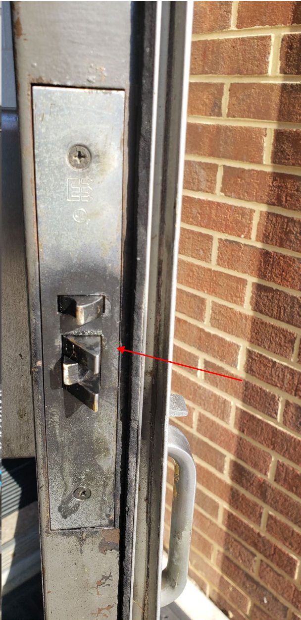
Figure 3 Lock mechanisms failing
